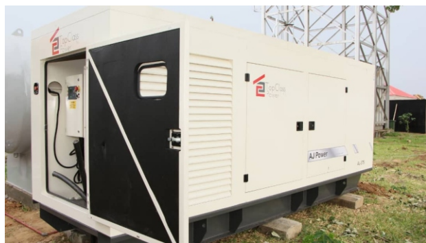
The newly installed 350KVA Perkins generator donated to the Isolation Centre by Mainstream Energy Solution Limited
