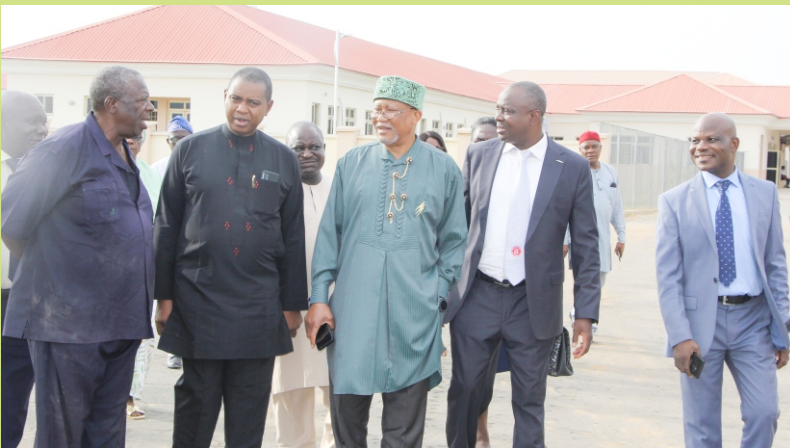
(From left to right) Engr. Meliga (Contractor), Dr. Bob Ukonu (CMAC), Dr. Sam Sam Jaja (Chairman, Board), Prof. B. A. Ekele (CMD), Mr. Ninfa Zwalbong (Director, Finance and Accounts) at a construction site.
